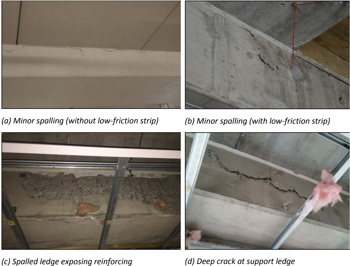
Figure 12: Examples of support ledge spalling
