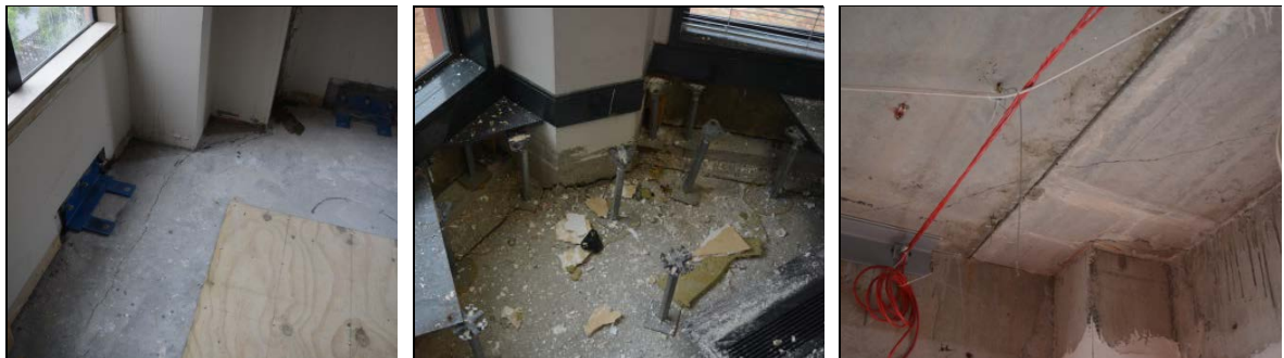
Figure 14: Damage in corners of floor plate – Single cracks
