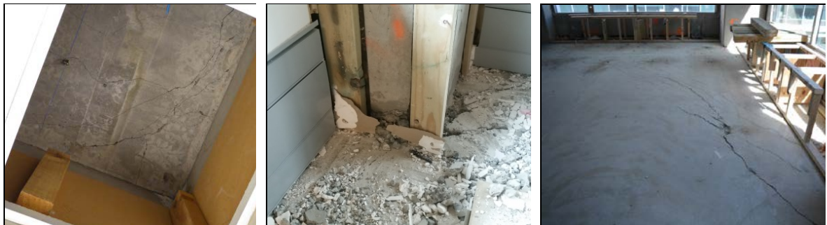
Figure 15: Damage in corners of floor plate – Significant cracking
