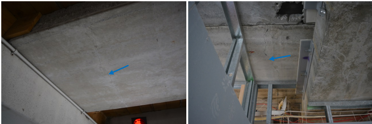
Figure 20: Transverse cracking of hollowcore away from support
