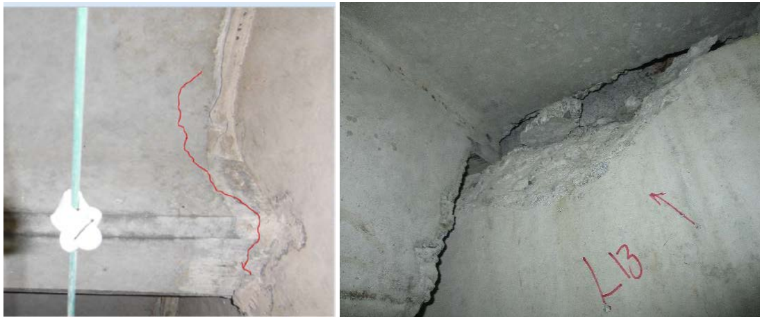
(a) Cracking of embedded tee rib (crack drawn for clarity)
