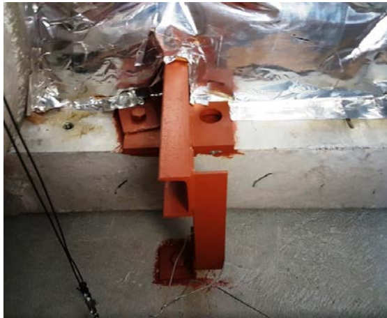
Figure 24: Precast cladding panel connection with fixing bolt not installed
