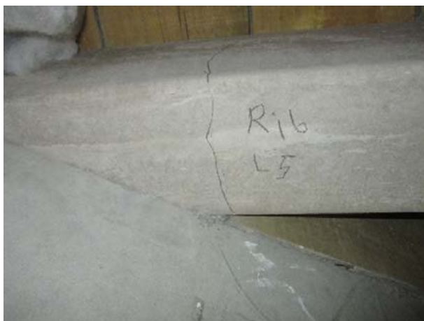
Figure 22: Transverse crack at end of rib (crack drawn for clarity)
