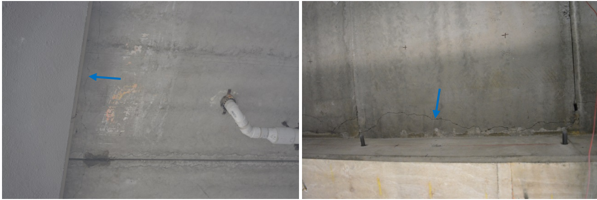
Figure 19: Transverse cracking of hollowcore close to support
