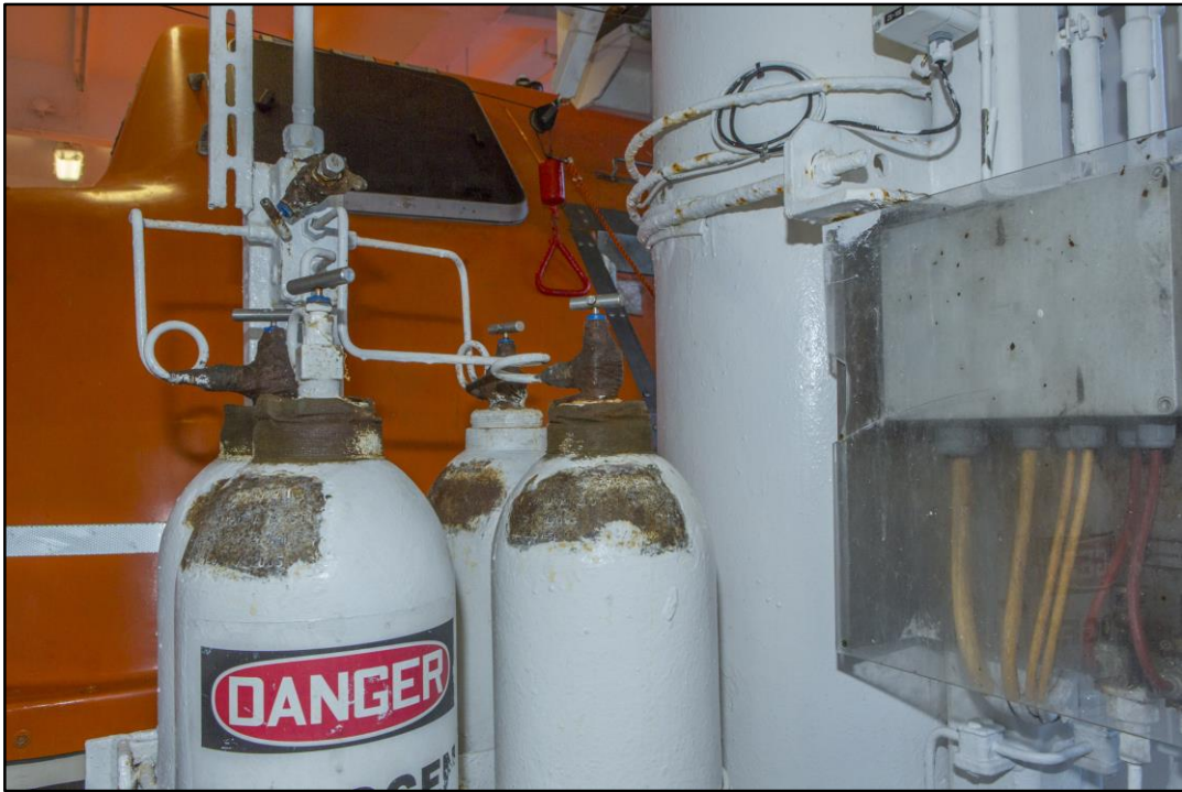
Figure 1 Typical four-cylinder installation on the Emerald Princess
