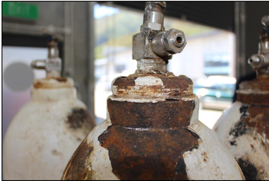
Figure 4 Significant corrosion around the top of other cylinder in the bank
