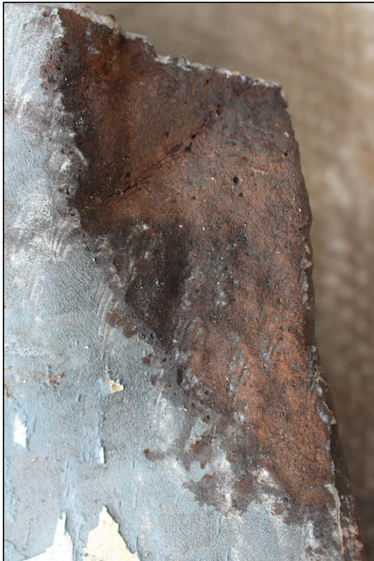
Figure 5 Significant corrosion at the point of failure
