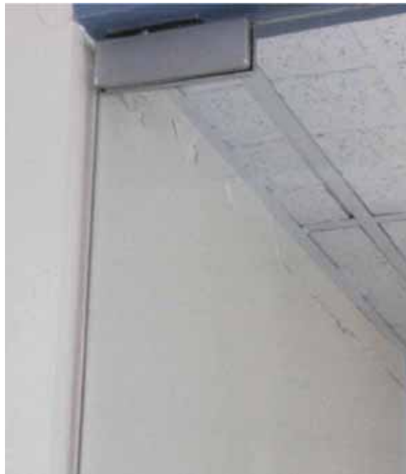
Figure 35: Horizontal crack along the ceiling at the north-eastern end of level 2 (source: Peter Brown)
