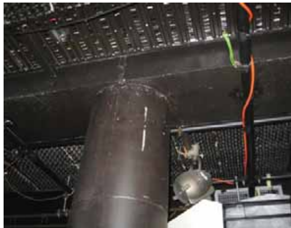
Figure 45: Internal beam-column connection under Level 2 with no evidence of damage (source: David Coatsworth)
