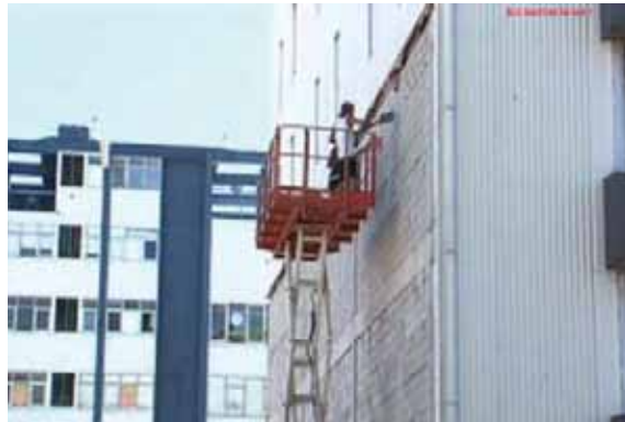
Figure 57: Leonard Fortune and co-worker on a scissor lift working on the western wall of the CTV building prior to the 22 February 2011 earthquake (source: Canterbury Television)
