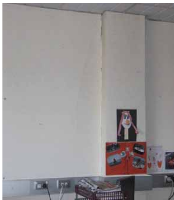
Figure 32: Vertical crack alongside pillar on western wall of level 2 (source: Peter Brown)
