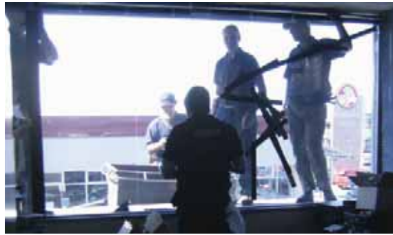
Figure 34: Replacement of a cracked window in the eastern wall on level 2 (source: Peter Brown)
