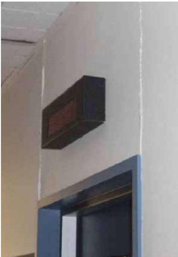
Figure 36: Two vertical cracks in an internal wall in the north-eastern end of level (source: Peter Brown)
