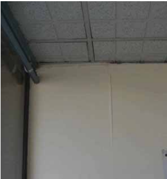
Figure 33: Two cracks in the north wall near the stair well on level 2 (source: Peter Brown)
