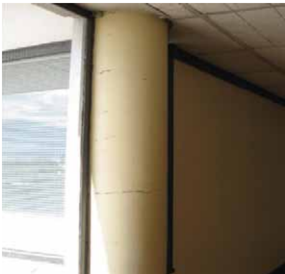
Figure 37: Cracked column C18 outside the lifts on level 6 (source: Leonard Pagan)
