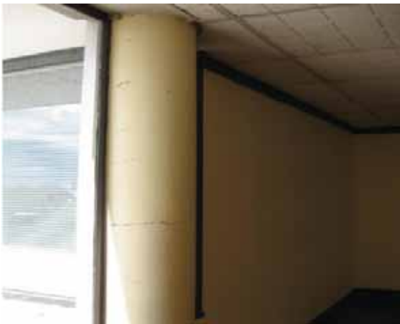
Figure 44: Cracking in column C18 adjacent to lift lobby (source: David Coatsworth)
