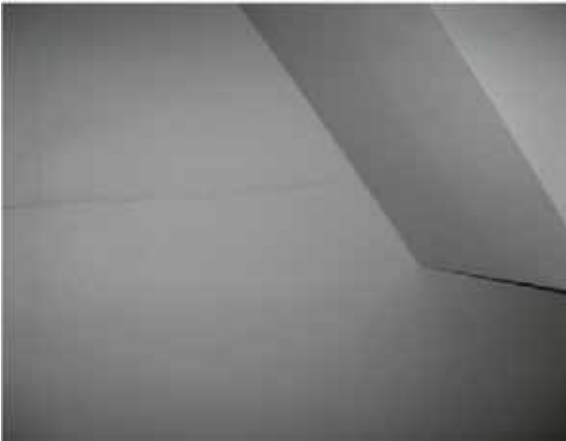
Figure 43: Cracking along construction connections in the north wall complex (source: David Coatsworth)
