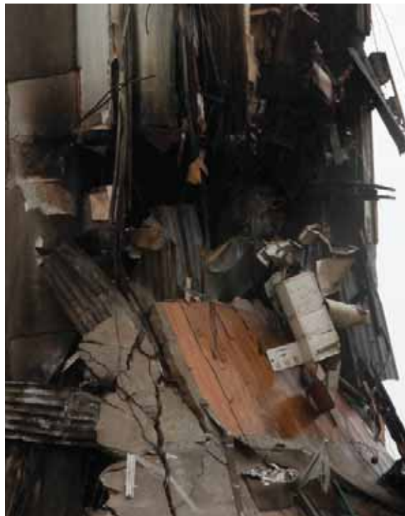
(b) Part of the north wall complex after the collapse
