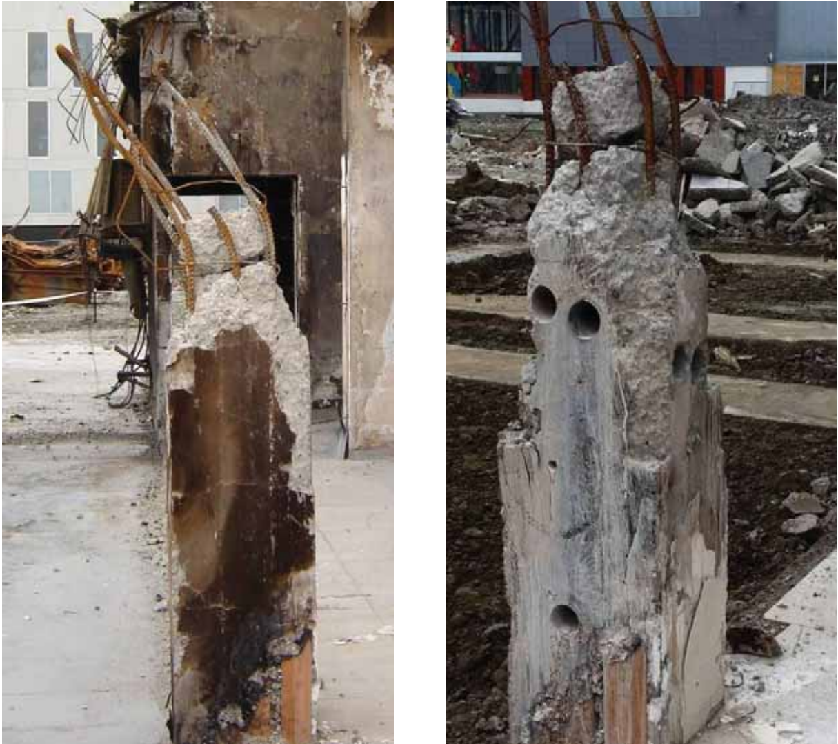
Figure 25: Concrete cores taken from column C18 on line 4, adjacent to wall D-E (source: Hyland/Smith report)
