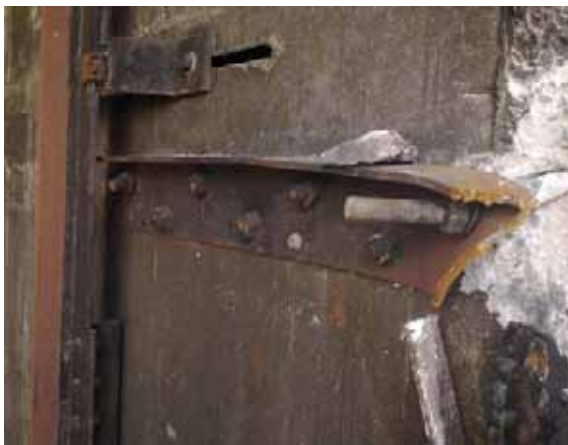
(c) A fractured drag bar on the wall on line D-E
