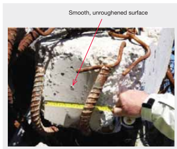
Figure 20: Smooth end of precast beam where it connected to circular columns (source: Dr Robert Heywood)
