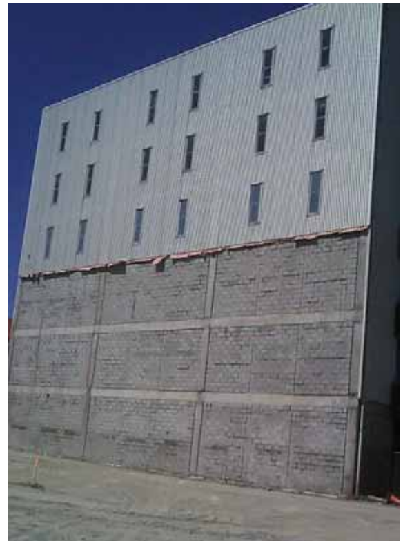
Figure 12: Photograph of the west wall after demolition of the building to the west, showing the block wall for the three lowest levels
