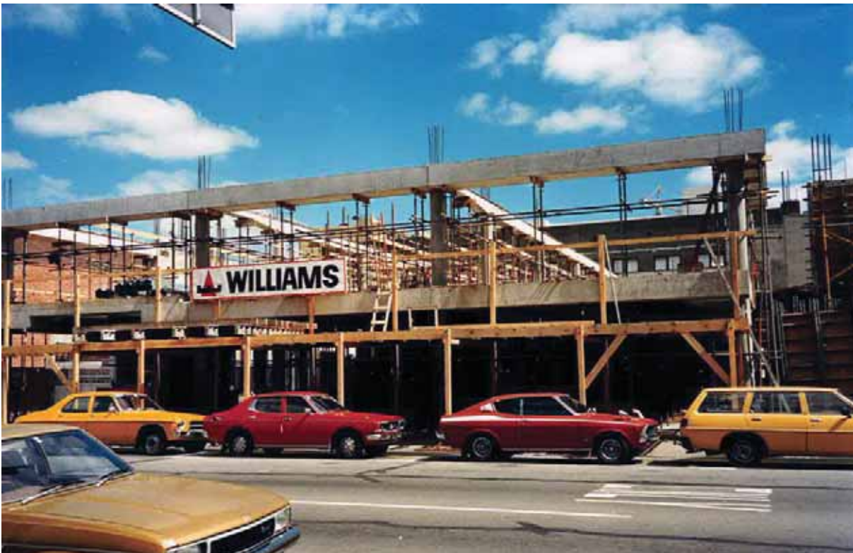
Figure 9: View of the building from Madras Street while under construction. The north wall complex is to the right. The beam structure can be seen, along with the external round columns. The upper beams are “shells” at this point and were filled with concrete at the same time as the floor was poured
