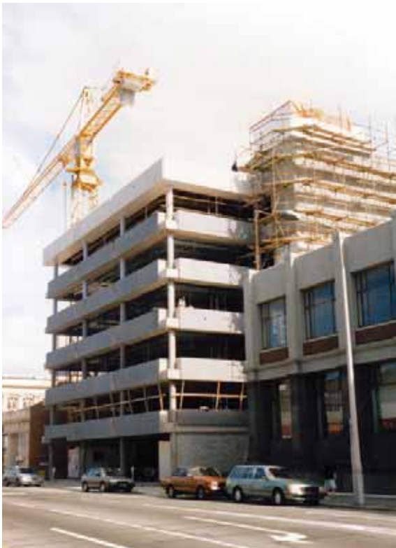
Figure 11: View from Madras Street. The spandrel panels are now fitted, and the north wall complex can be seen covered in scaffolding
