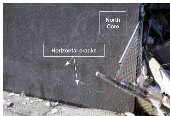
(b) Cracking in northern face, western end (source: Robert Heywood)
