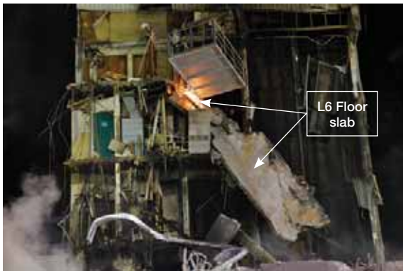
(a) Detachment of floors at levels 4, 5 and 6
