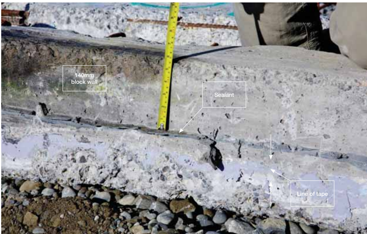
Figure 68: Sealant on a remnant of the western wall (source: Robert Heywood)
