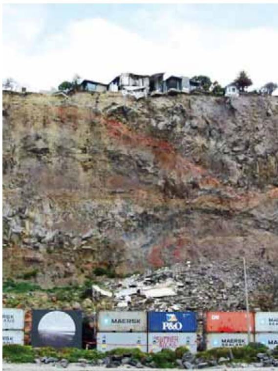
Figure 7: Collapsing rocks in the suburb of Sumner caused houses to fall down the cliff. A row of shipping containers was installed to protect the busy road below from danger (source: Flickr/newtown graffiti)
