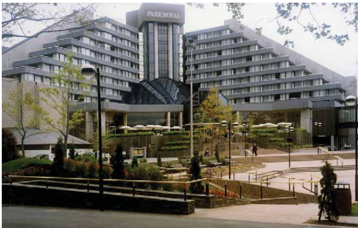
Figure 13: The Crowne Plaza Hotel, formerly the Park Royal Hotel, was damaged by the earthquakes and demolished in 2012 (source: Gudrun Gisella)
