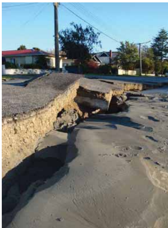
Figure 8: Road damage caused by the earthquakes (source: Michael Campbell)
